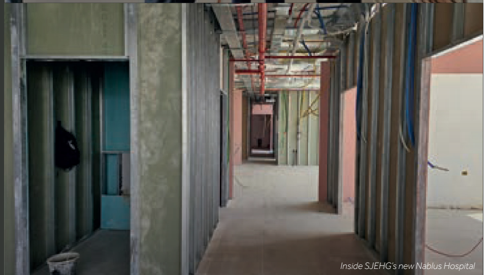
CEO Dr Ahmad Ma'ali and Facilities Manager Ahmad Awadallah pictured on site with the engineer overseeing the work
