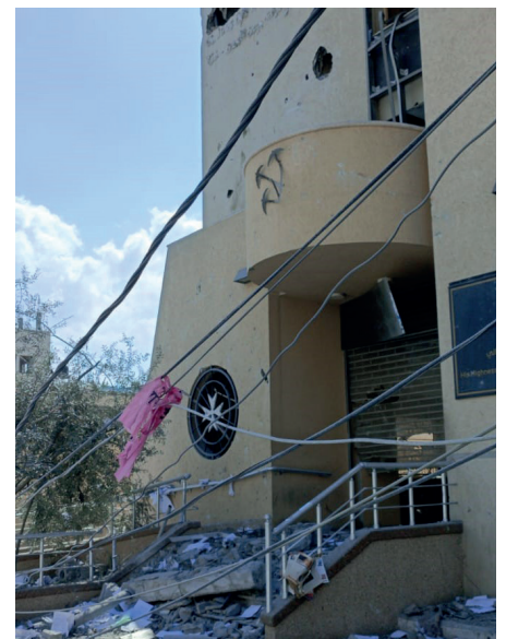
SJEGH's hospital in Gaza City having sustained collateral bomb damage
